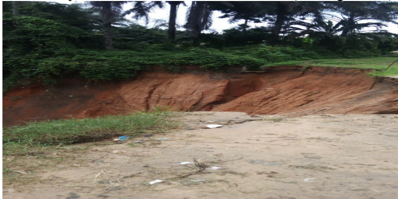
Picture 2: Failed portion of road site at Ariam-Usaka ring (Amaegbu-Ariam) road.
